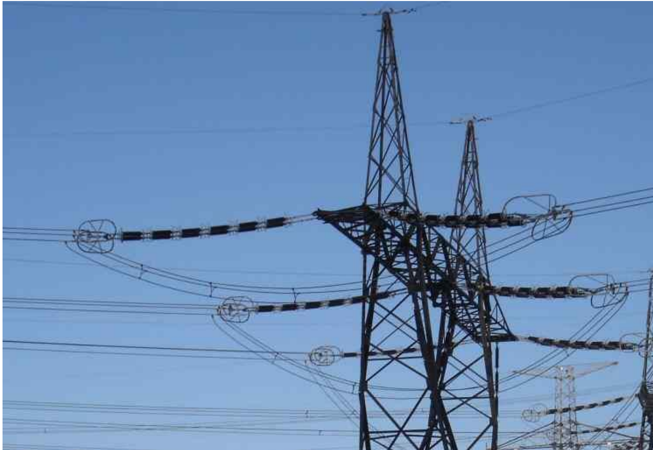
Dead-end insulator string
