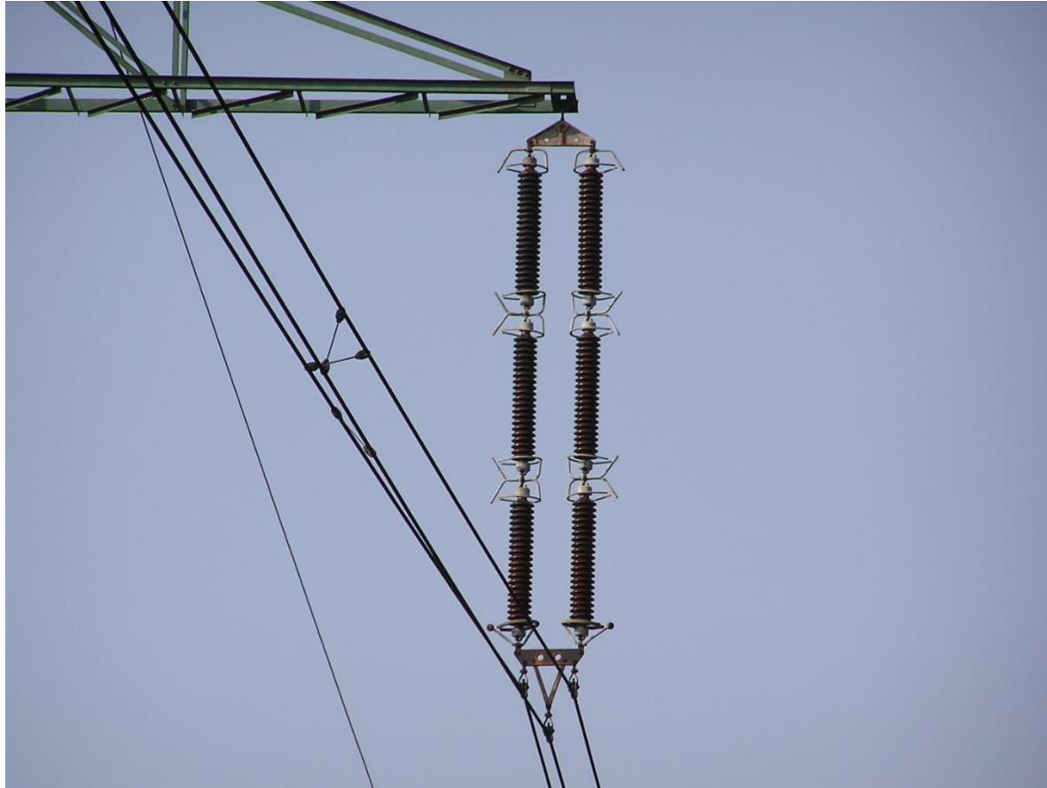
Suspension insulator string
